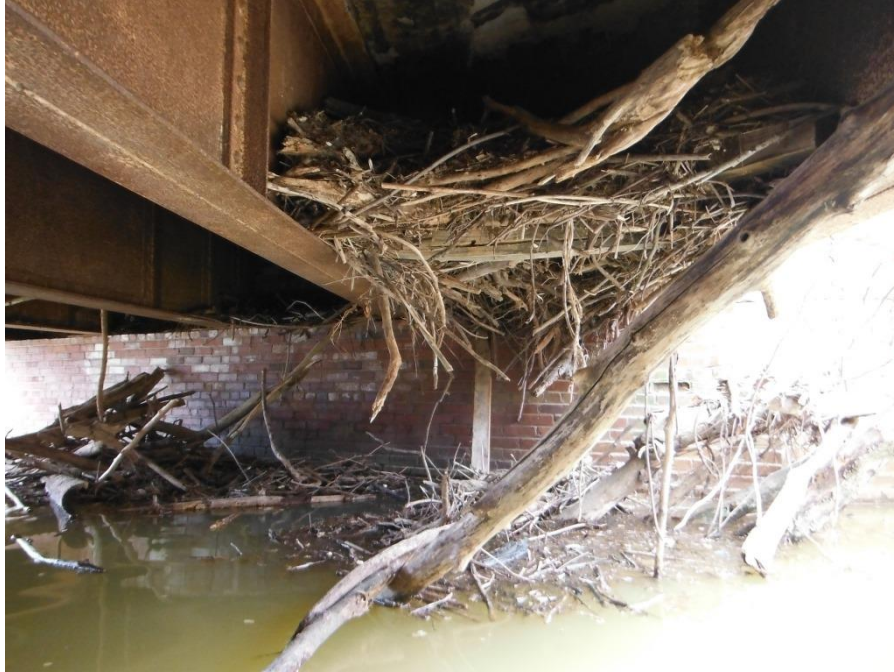
Photo 19: Debris between girders and at west abutment
