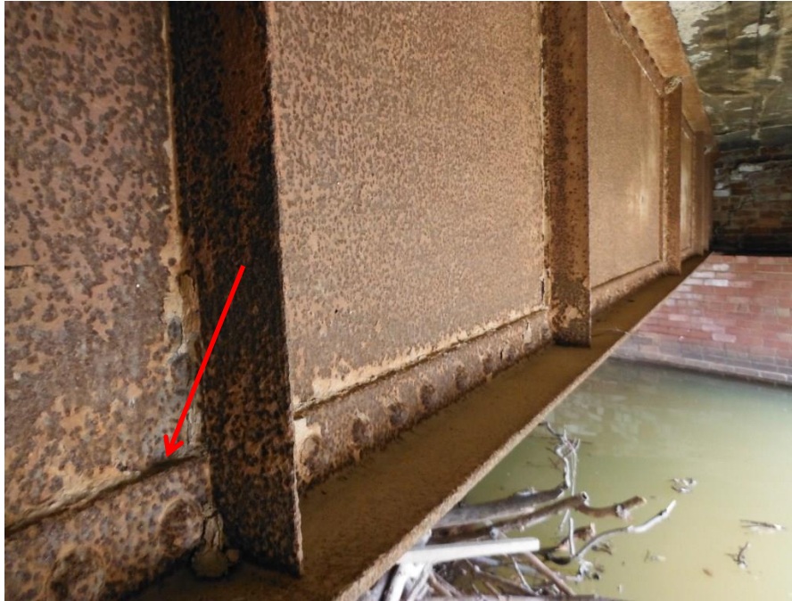
Photo 9: Surface rust and pitting on girder #4, looking from west abutment; Note pack rust between web plate and bottom flange angle
