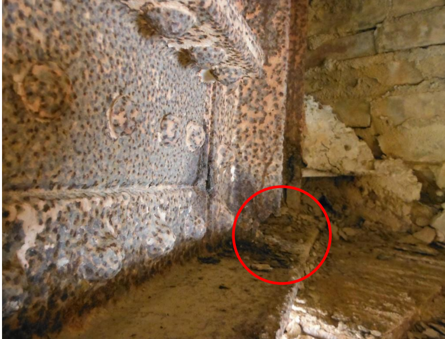
Photo 11: Hole in base of girder #1 bearing stiffener at east abutment, south side of girder
