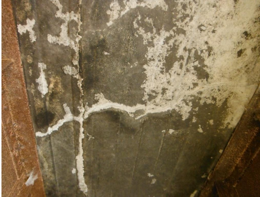
Photo 5: Transverse crack on bottom of deck near east abutment between girders #4 & #5
