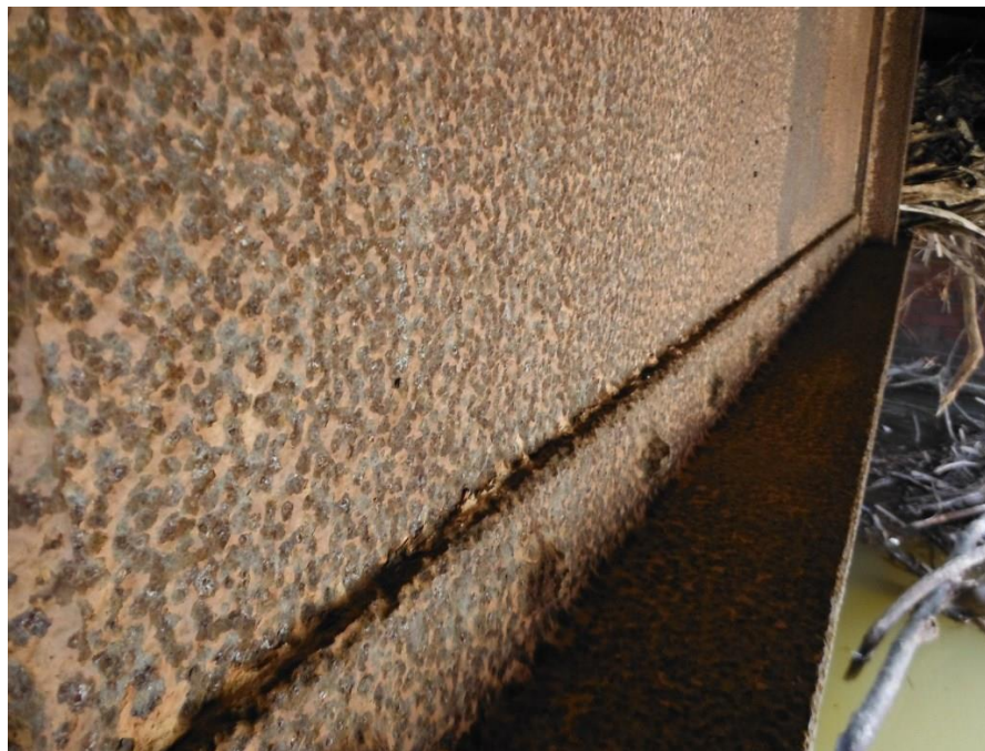
Photo 10: Pack rust between girder #2 web plate and bottom flange angle, looking from east abutment
