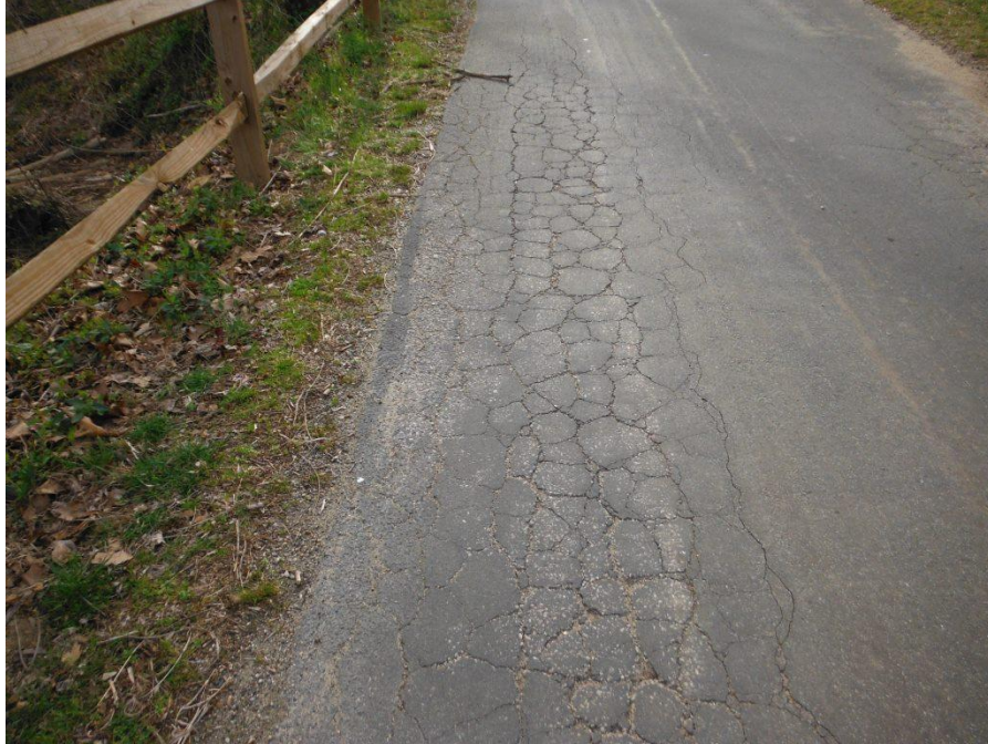
Photo 3: Map cracking in asphalt wearing surface and west approach pavement
