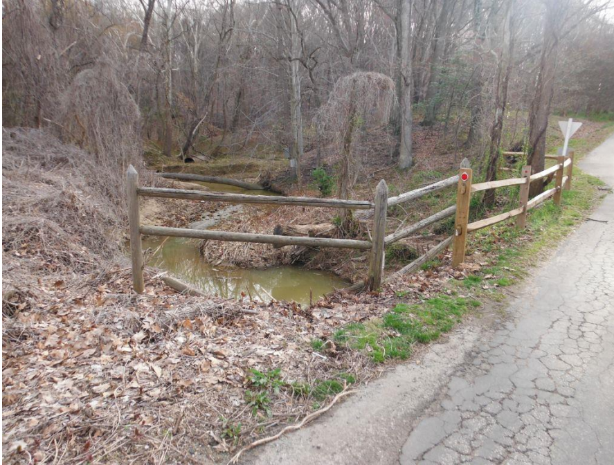
Photo 7: Old deteriorated timber railing remains at northwest corner
