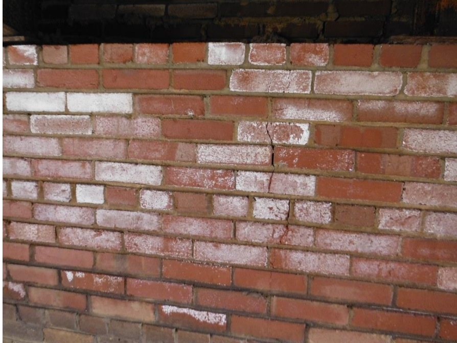
Photo 17: Vertical crack in bricks and mortar joints on east abutment breastwall between girders #3 & #4
