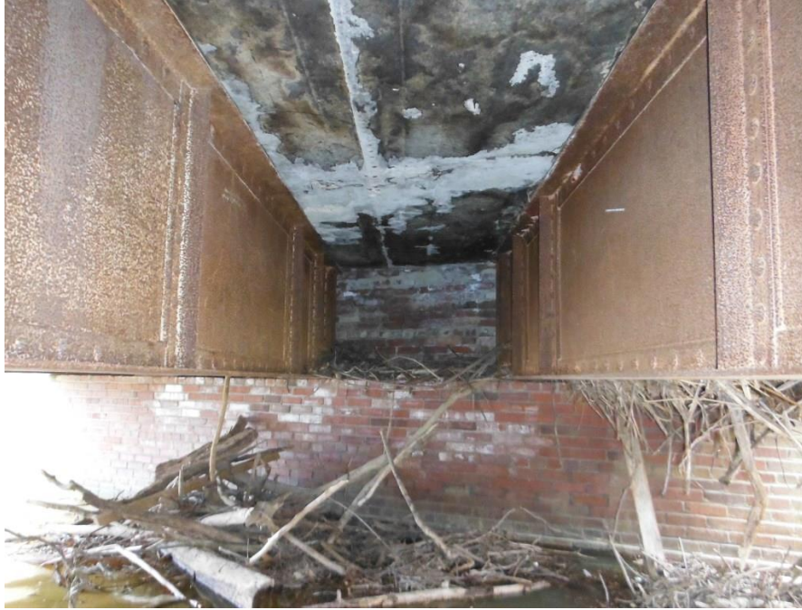
Photo 15: Debris on west abutment seat between girders #2 & #3
