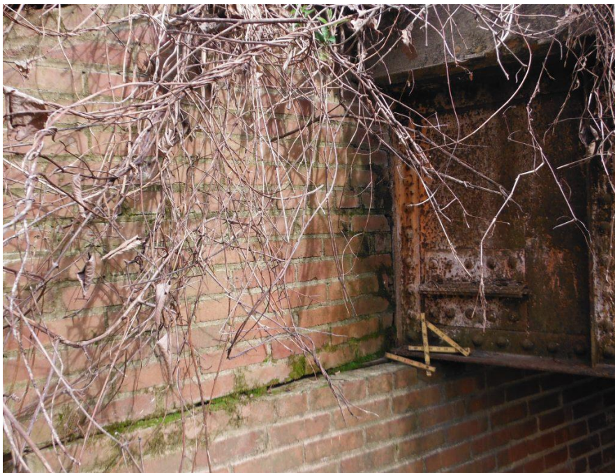
Photo 12: Open joint at seat level with lateral movement of southwest wingwall
