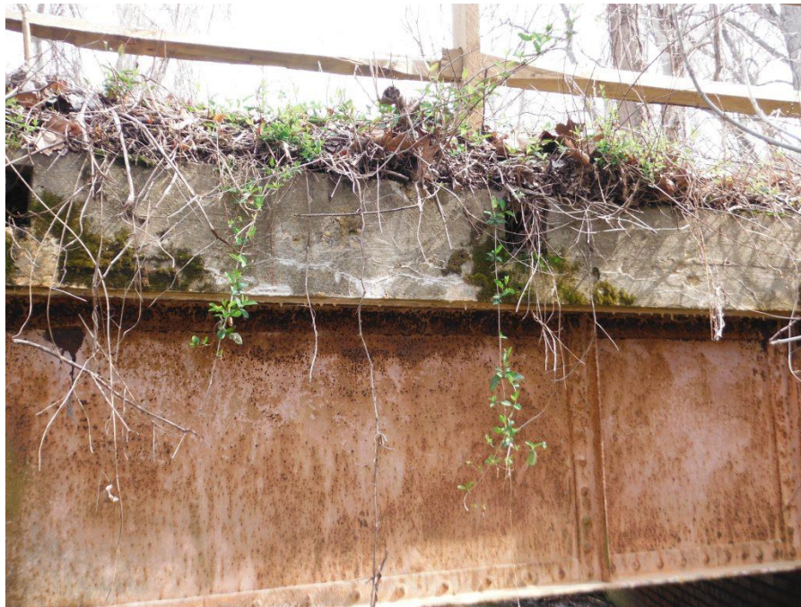
Photo 4: Horizontal cracking with efflorescence on south fascia of deck
