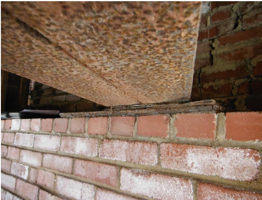
Photo 8: Rust and pack rust on girder 4 bearing plate at east abutment
