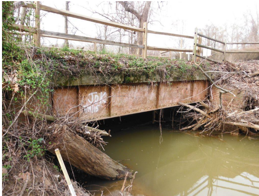
Photo 20: Debris in upstream channel in front of wingwalls
