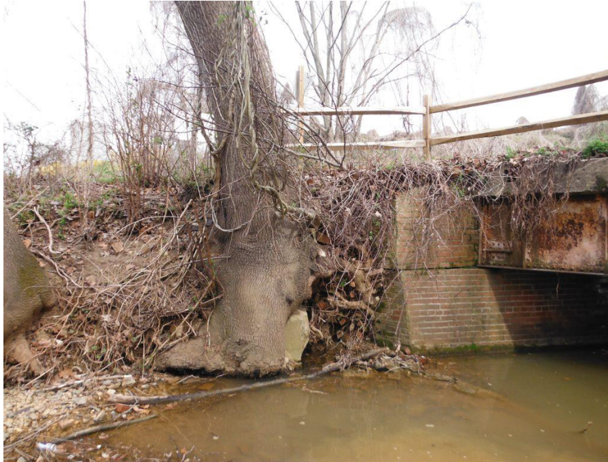
Photo 13: Deteriorated end of southwest wingwall at location where tree has fallen
