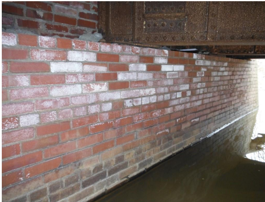
Photo 16: General view of east abutment; Note staining on breastwall near waterline
