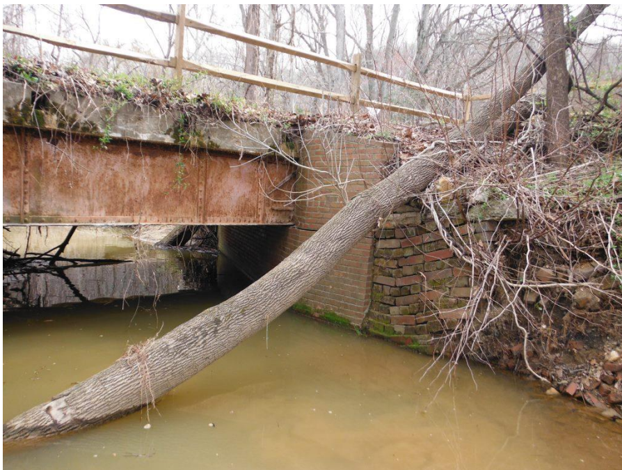
Photo 18: Tree fallen across downstream channel onto southeast wingwall; Note tree was previously in front of southwest wingwall
