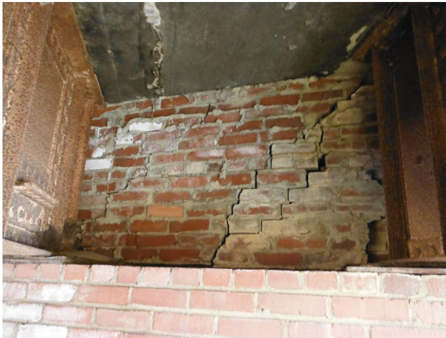
Photo 14: Diagonal crack in east abutment backwall between girders #4 & #5
