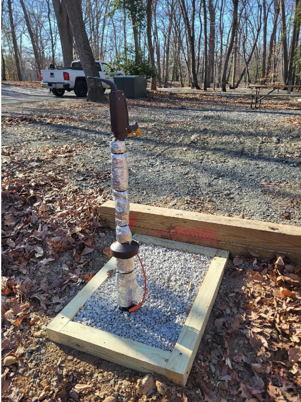
1. Hydrant foundation box, heat tape & insulation
