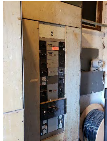
E-2: Existing Panel MDP and Meter
